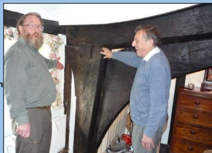
Right a rare solid brace between baypost and tie beam in a Wealden style building with jettied bays either side of the open hall .
